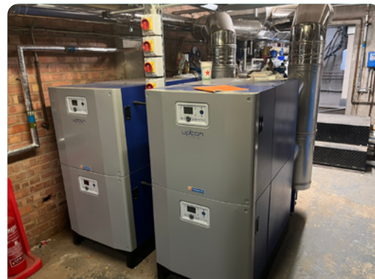
Undersoil heating boiler
