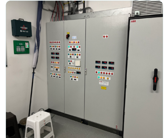
VV control panel
