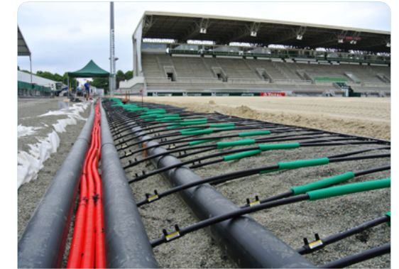
Undersoil heating system
